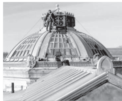
Bangor Public Library's leaking roof.
